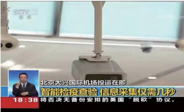
Application at Beijing Daxing International Airport
